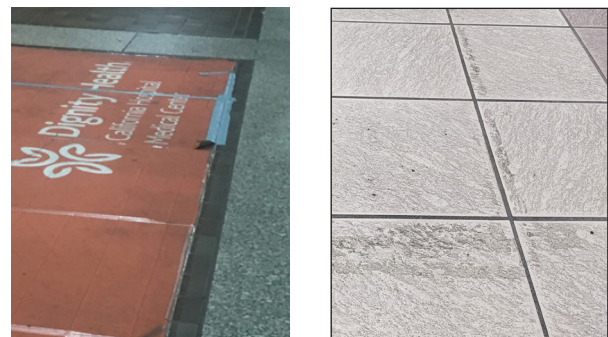
Figure 1-5 Poor quality adhesive floor decal (left; 7th Street/Metro Center Station) and damage left behind, known as "ghosting" (right; Union Station).
