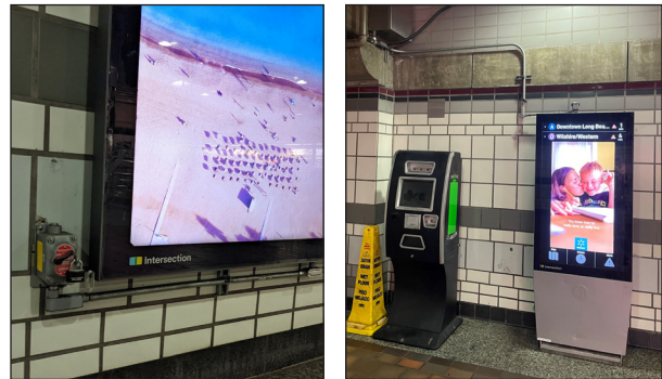
Figure 1-1 Poorly integrated electronic information displays, which create eyesores and potentially present cleaning, maintenance, vandalism and safety issues (7th Street/Metro Center Station).
