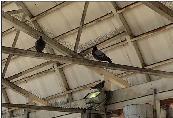
Figure 2-1 Ineffective deterrents at Harbor Freeway Station.
